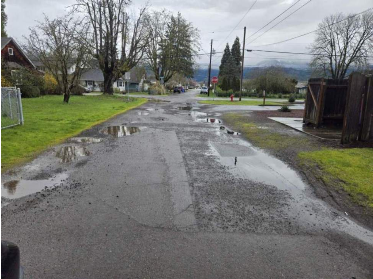
Figure 4: E. McKenzie St. between N. Coleman St. and N. Skinner St. showing degraded pavement and resulting ponded water after a mild rainfall event, looking east.
