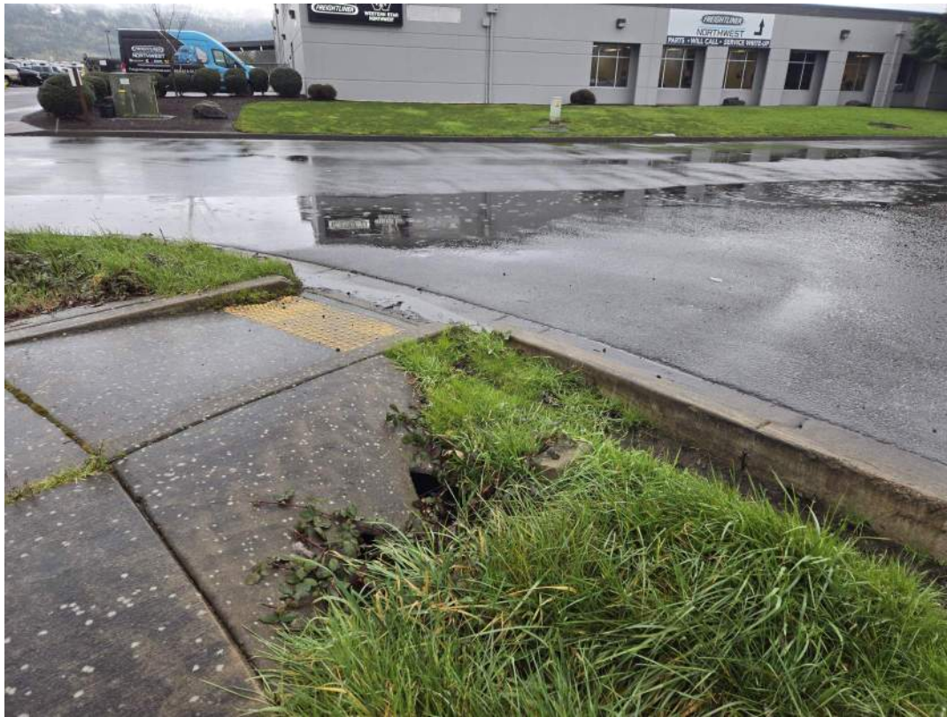
Figure 92: Coburg Industrial Way overgrown culvert in 2024.
