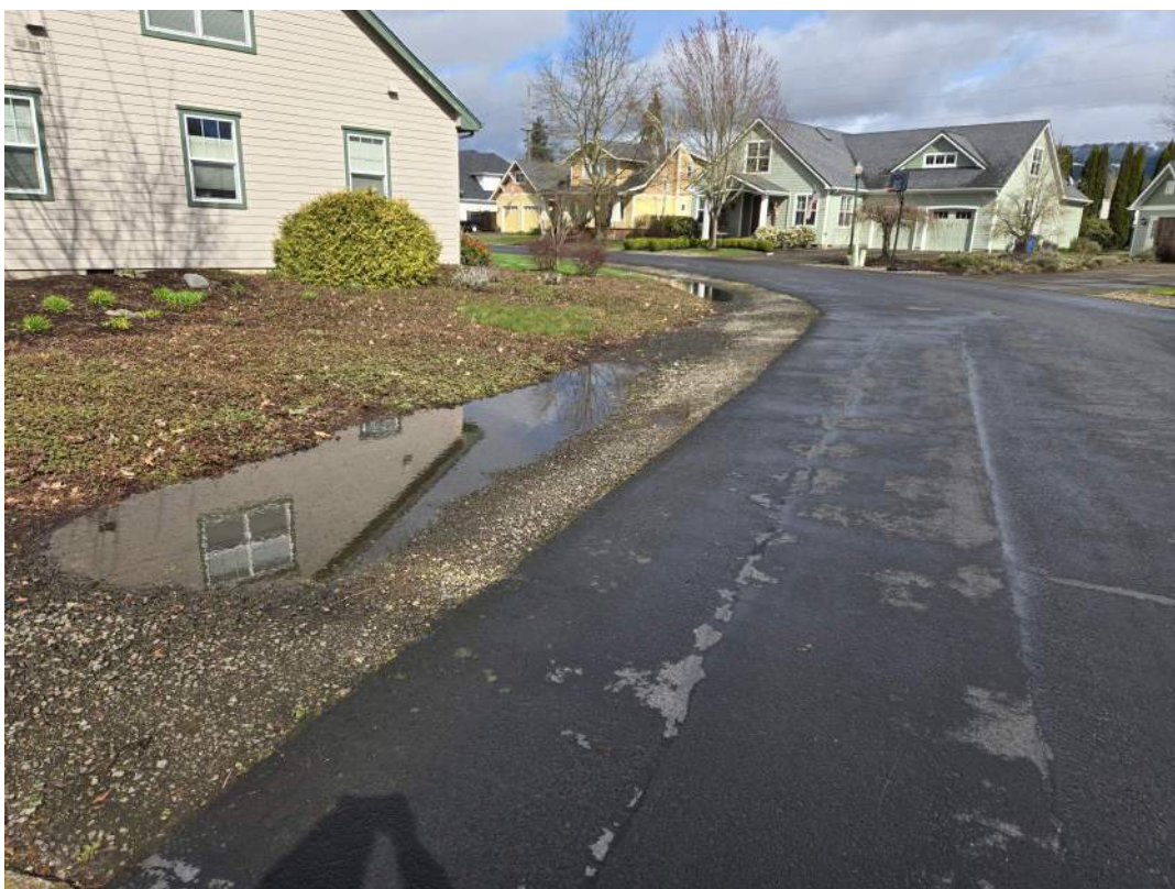
Figure 87: Austin St. infiltration deficiency in 2024.
