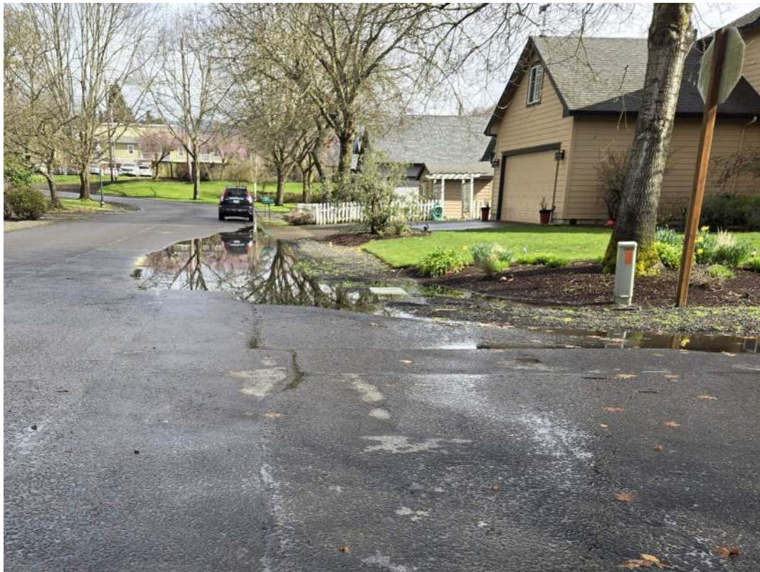
Figure 86: Abby Rd. and W. McKenzie St. standing water in 2024.
