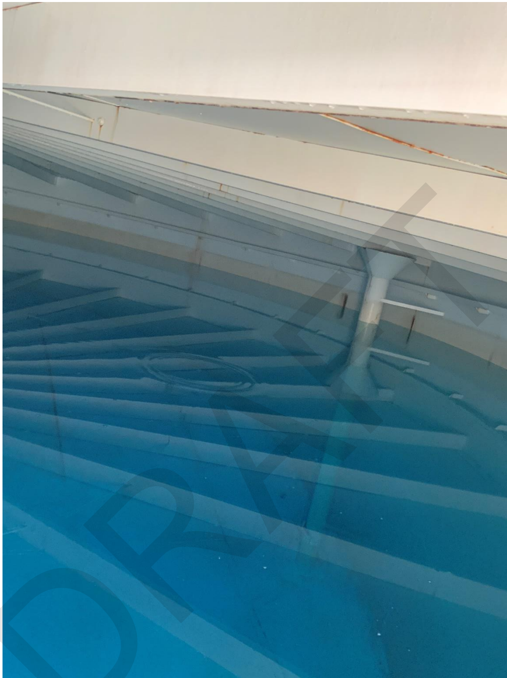
Photo 24 – Tank Interior Overflow Pipe
