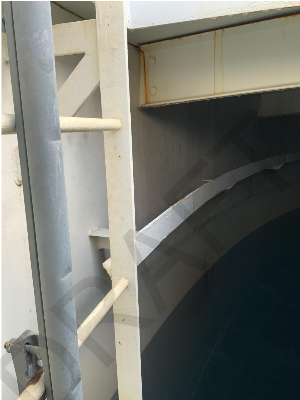
Photo 26 – Tank Interior Roof Framing Corrosion
