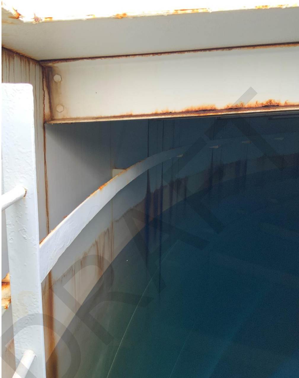
Photo 13 – Tank Interior Roof Framing Corrosion
