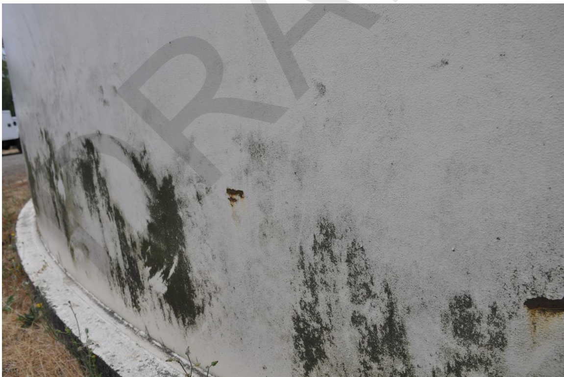
Photo 19 – Tank Exterior Coating Deterioration
