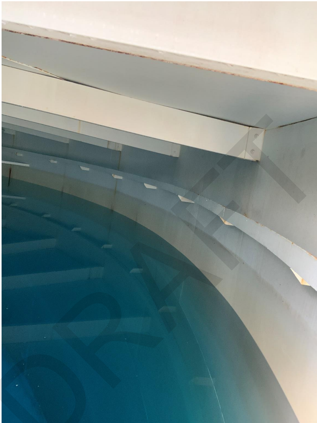
Photo 25 – Tank Interior Roof Framing Corrosion
