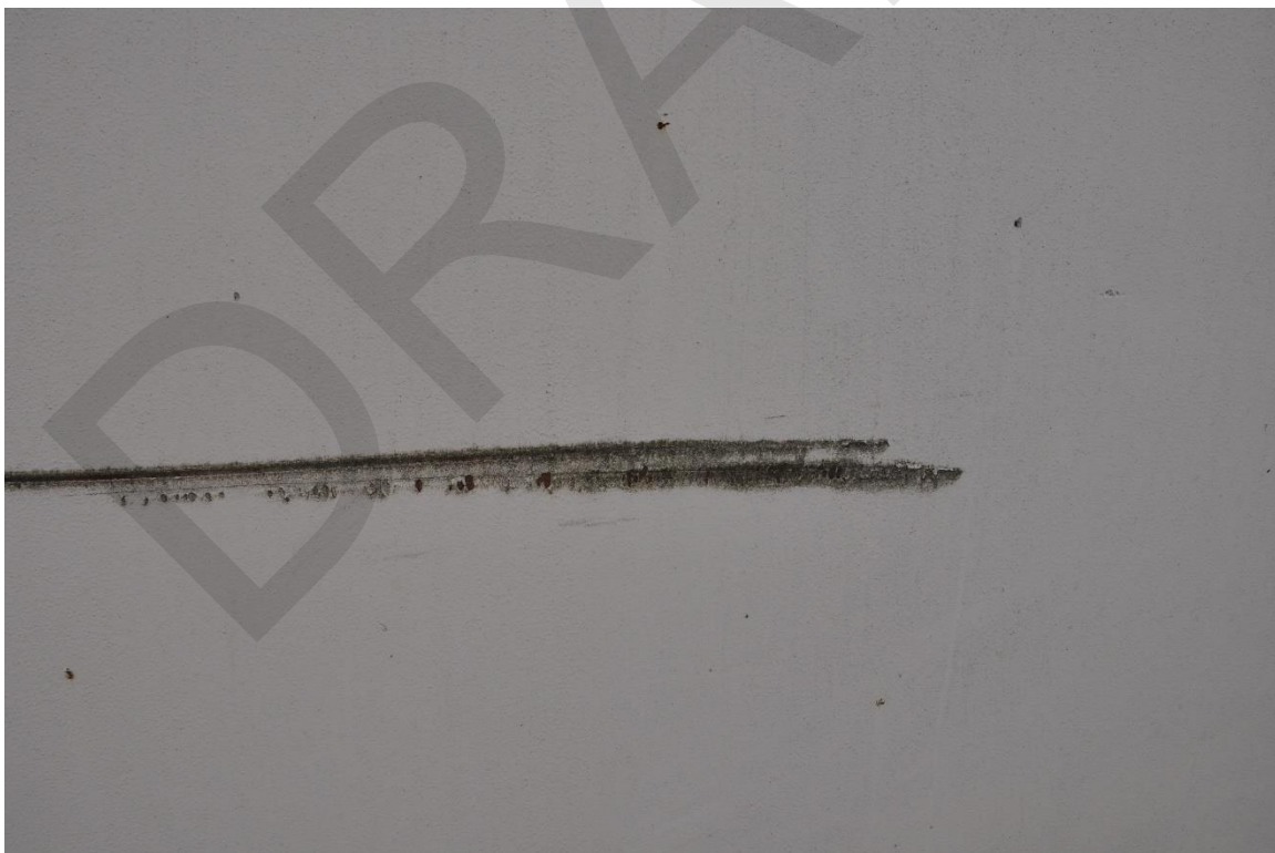
Photo 6 – Tank Exterior Coating Deterioration
