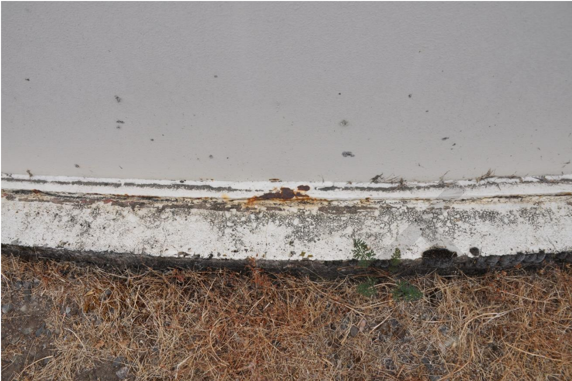
Photo 20 – Tank Exterior Coating Deterioration
