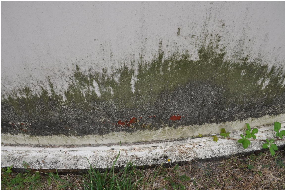
Photo 7 – Tank Exterior Coating Deterioration
