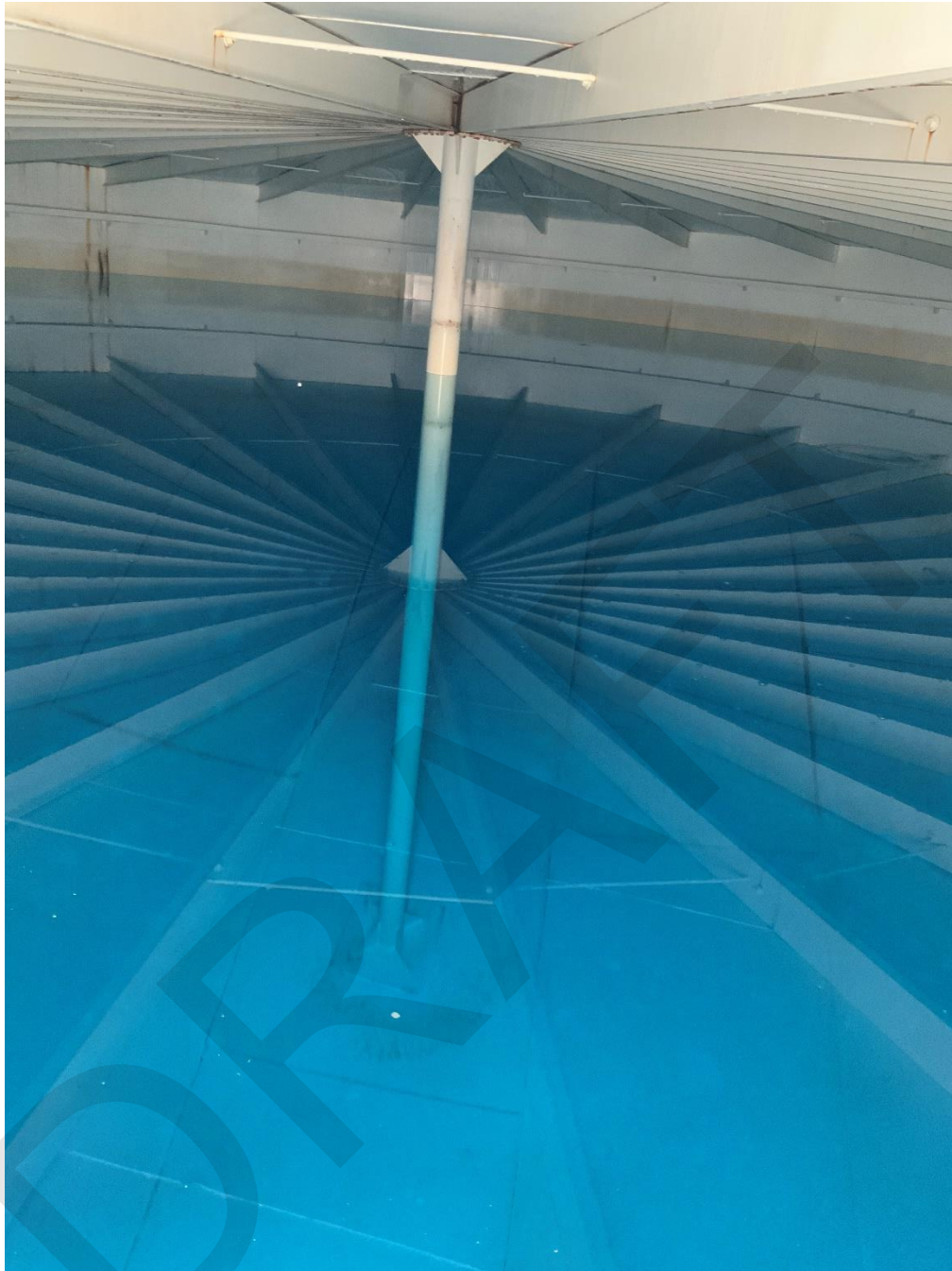
Photo 22 – Tank Interior Center Column
