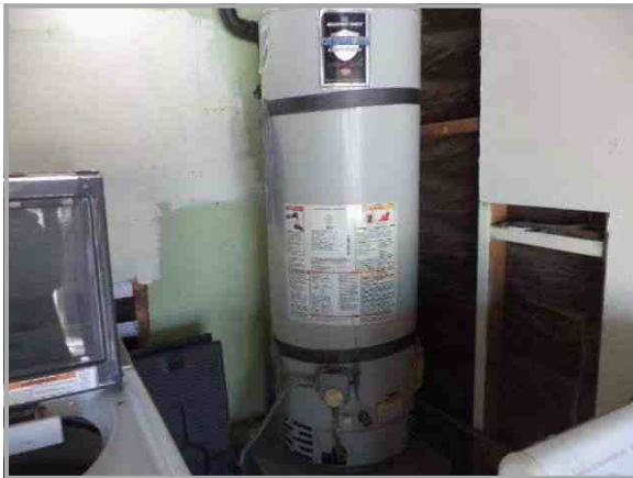
Earthquake strapped water heater
