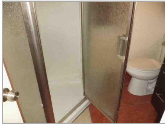
hall bathroom shower
