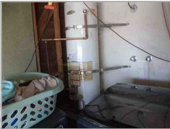
Earthquake strapped water heater
