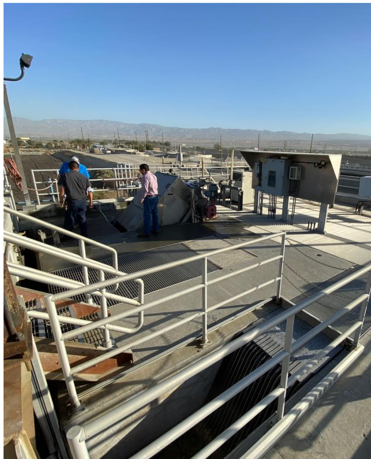
Figure – 1: Site Photo Showing: Existing Bar Screen; Existing Secondary Channel (not is use) and Manual Bypass Channel
