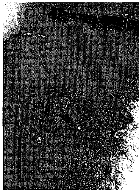
Popcorn ceiling debris
