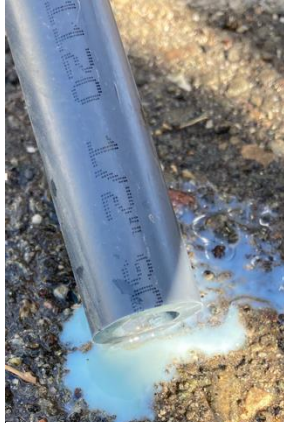
Figure 1. Tin and chromium residuals accumulated in pipe following pilot testing of stannous chloride without filtration in Dixon, CA (2023).
