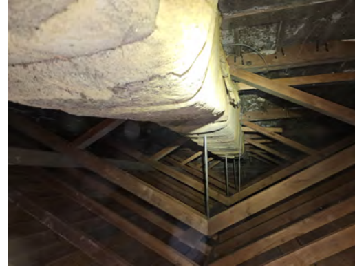
No as-built drawings & data for building structural elements between diagonals and chord
