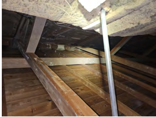
Roof trusses have no positive connections required by code
