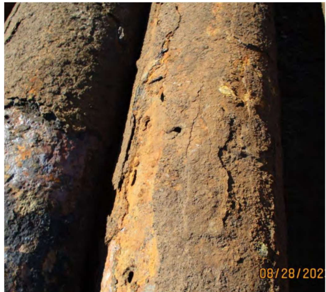
Figure 1: Severe corrosion and oxidation on Well 16 pump column pipe.
