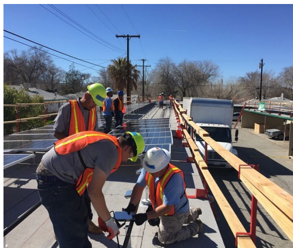
◆ Figure 11: Transform Fresno Solar Installation
