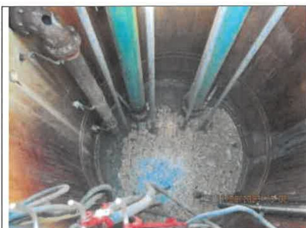
Photo 17: A photo of the wet well at Pump Station No. 3 showing a FOG mat, rags on the pipes, corrosion, and staining on the walls.
