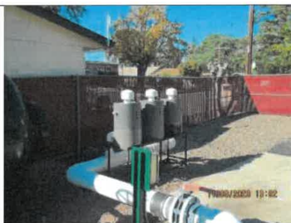
Photo 18: A photo of the carbon odor control system at Pump Station No. 3.
