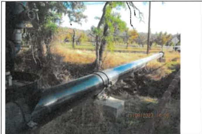
Photo 30: A photo of the force main aerial crossing located at the intersection of Rusmey Road and Pamela Lane with no secondary encasement.
