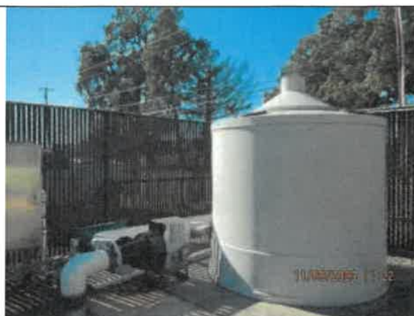
Photo 8: A photo of the carbon filter system at Pump Station No. 1 for odor control.
