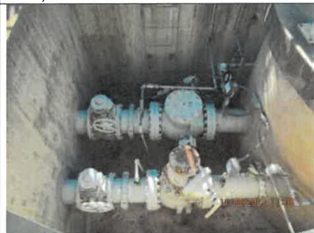
Photo 5: A photo of the one of the uncovered dry wells with minimal debris and paint chippings.
