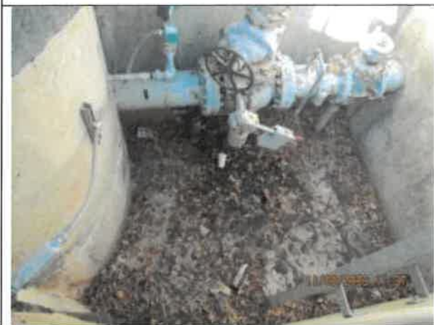
Photo 11: A photo of the uncovered north dry well at Pump Station No. 2 showing debris and minor trash.
