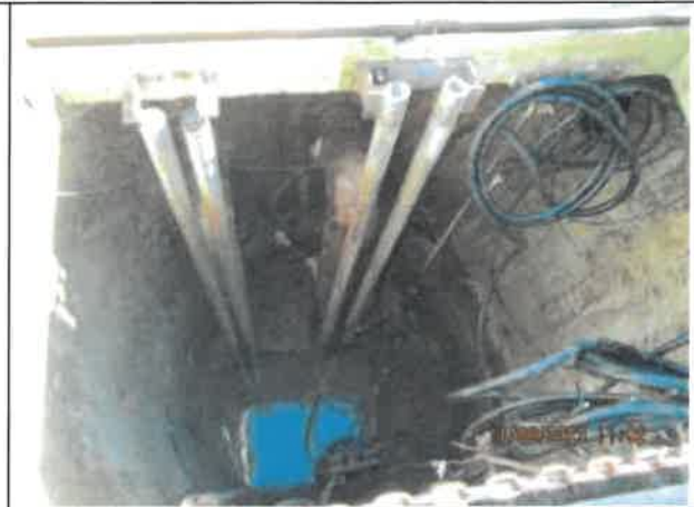
Photo 2: A photo of the wet well on the south side of Pump Station No. 1 with minor FOG, rags, and corrosion.
