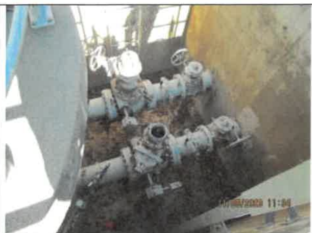
Photo 10: A photo of the uncovered south dry well at Pump Station No. 2 showing debris and a missing cap on one of the connections.
