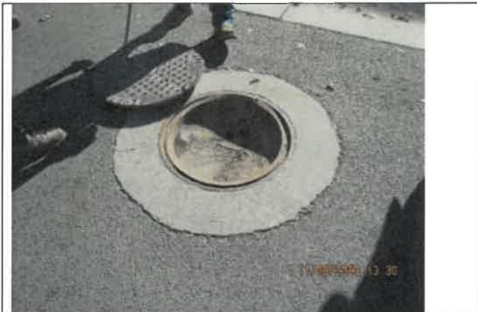
Photo 25: A photo on the manhole located in front of 6925 Meadowbrook Drive with a manhole barrier lid and cracking in the concrete around the manhole.
