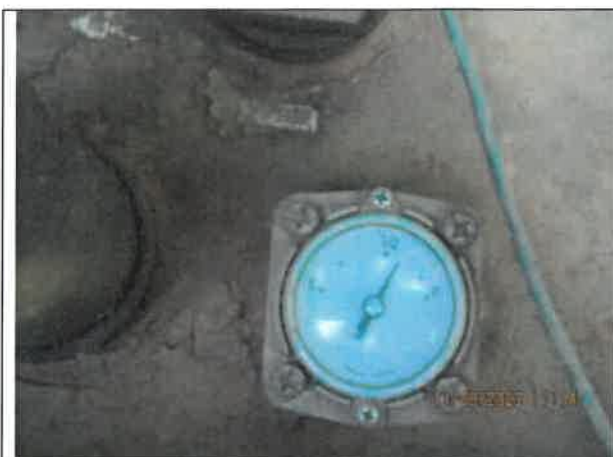
Photo 7: A photo of the fuel level of the generator at Pump Station No. 1 showing over 50 percent full.
