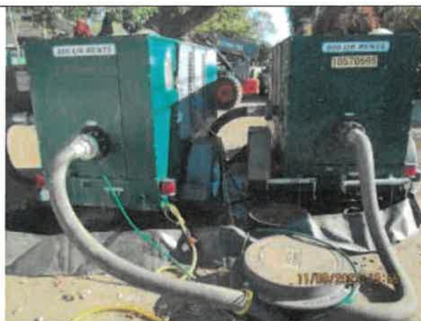
Photo 29: A photo of the portable bypass system being used while Pump Station No. 6 is under construction.
