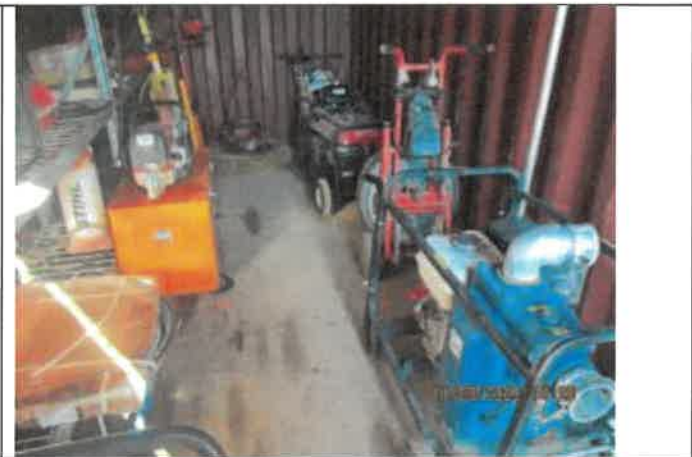
Photo 33: A photo of the portable generators at the utility yard.
