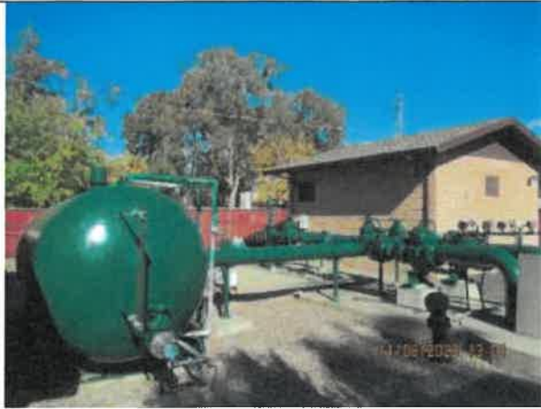
Photo 19: A photo of the recently painted aboveground pumps and piping system at Pump Station No. 3.
