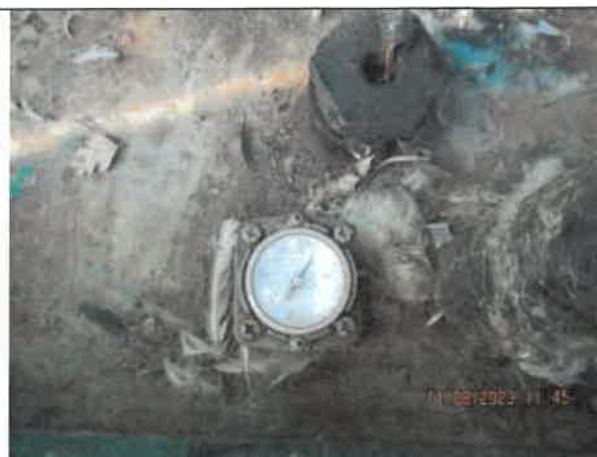
Photo 16: A photo of the fuel level of the generator at Pump Station No. 2 showing the fuel level to be over half full.
