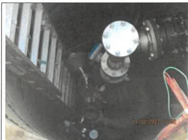
Photo 28: A photo of the direct in-line pumping system being put into place at Pump Station No. 6.
