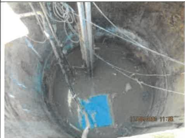
Photo 13: A photo of the north wet well at Pump Station No. 2 showing minor debris, trash, and staining on the walls.
