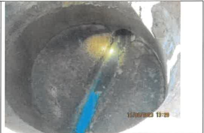
Photo 26: A photo on the manhole located in front of 6925 Meadowbrook Drive with a vertical crack in the manhole barrier and no flow in the channel.
