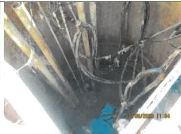
Photo 3: A photo of the wet well on the north side of Pump Station No. 1 with rags, minor FOG, and minor corrosion.
