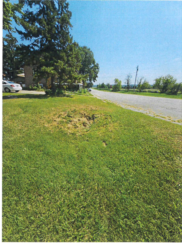
▲ 6 – West End of Winnegamie Drive Culvert (North Side) Upstream End of Bennett’s Auto Culvert
