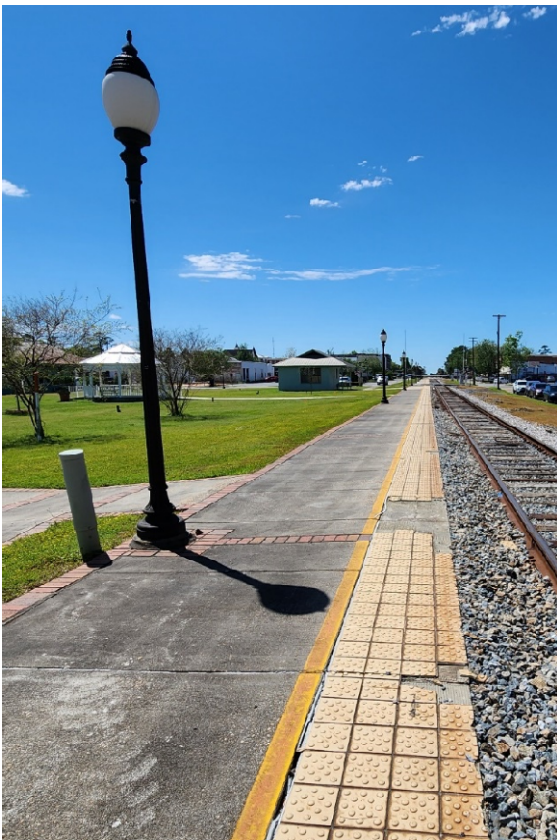
Photo 27. Pavements where tiles or bricks have been introduced represent tripping hazards to pedestrians when maintenance is lacking.
