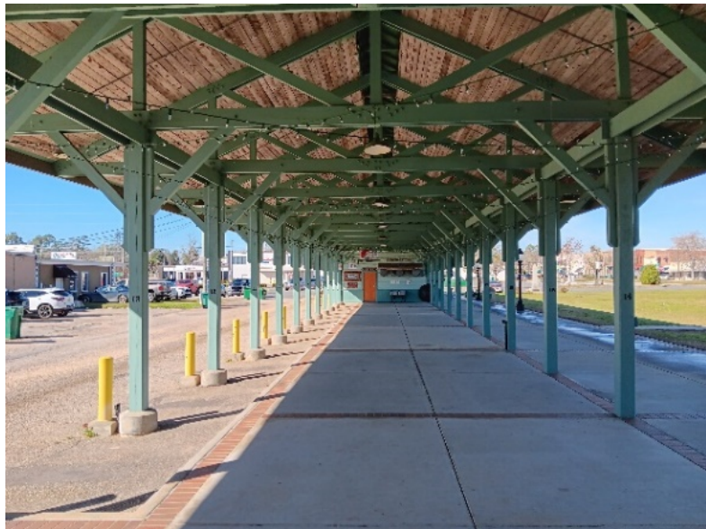
Photo 13. Architectural features of the re-created depot structure, home of the Chipley Farmer's Market.
