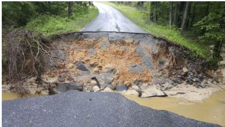
Chalk Level Road near South Hill after heavy rains in May, 2018. Photo credit: SoVaNow.com
