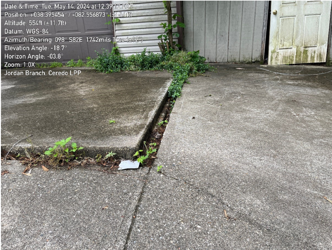
Figure 4. Concrete slab is displaced.
