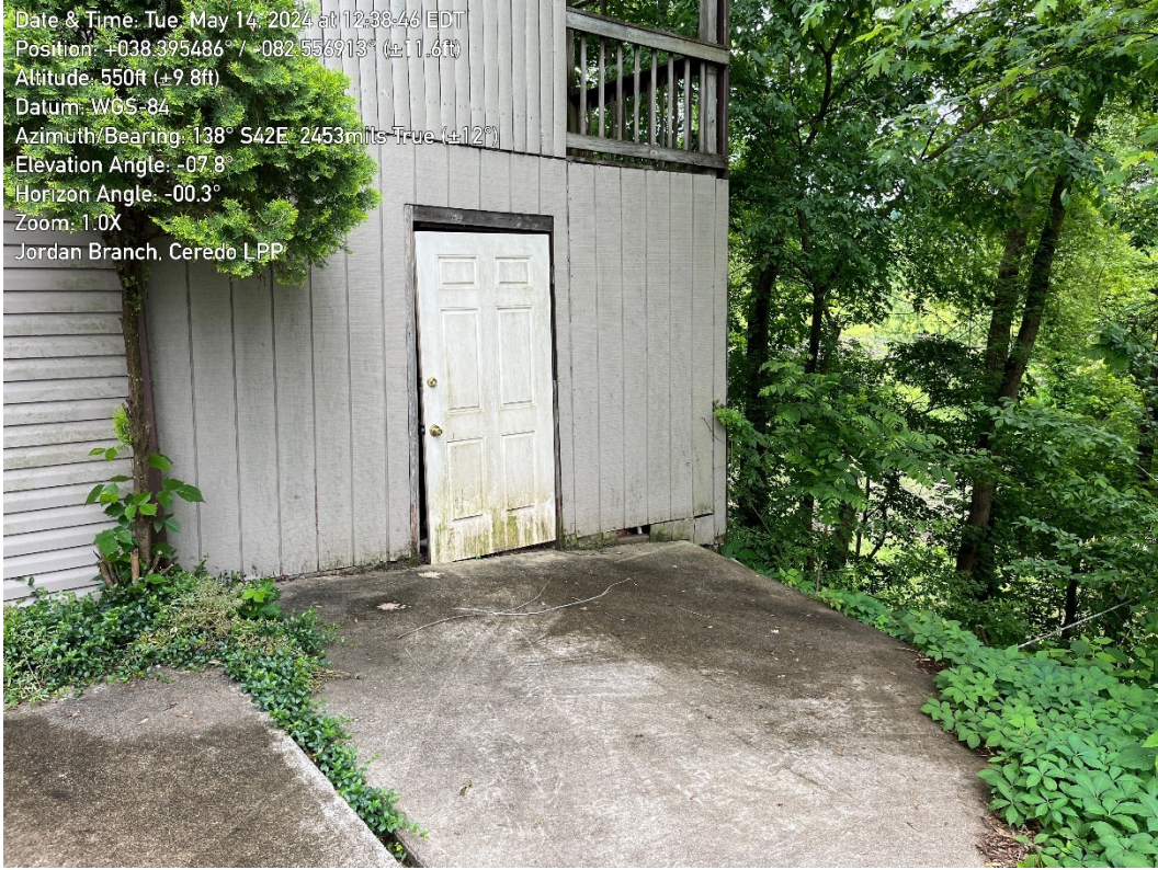
Figure 3. Concrete slab is tilted from left-to-right.
