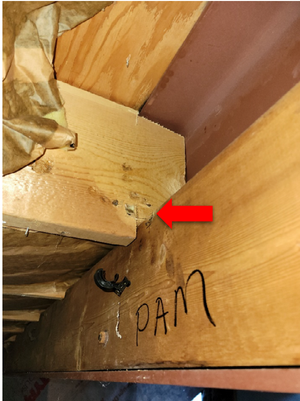
Notched Joist at Steel Beam
