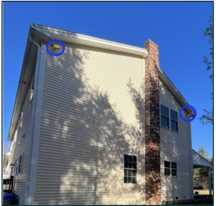
Side of structure: 2 floodlights.
