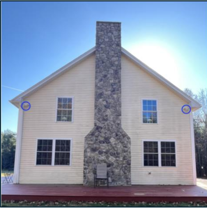
Side of structure: 2 floodlights.
