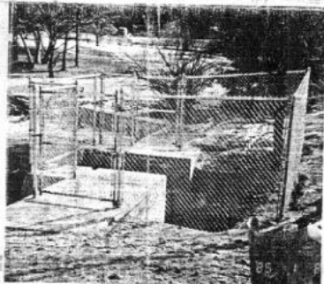
ALL REPAIRED — Dingley Dam today is all repaired and protected by high wire fence.
