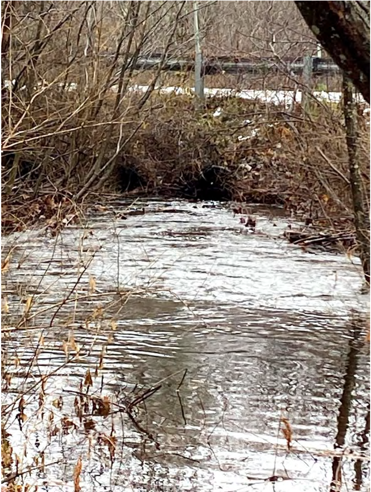
High Water – Looking at Culvert Inlet from Davis Brook Road (taken December 11, 2023)
