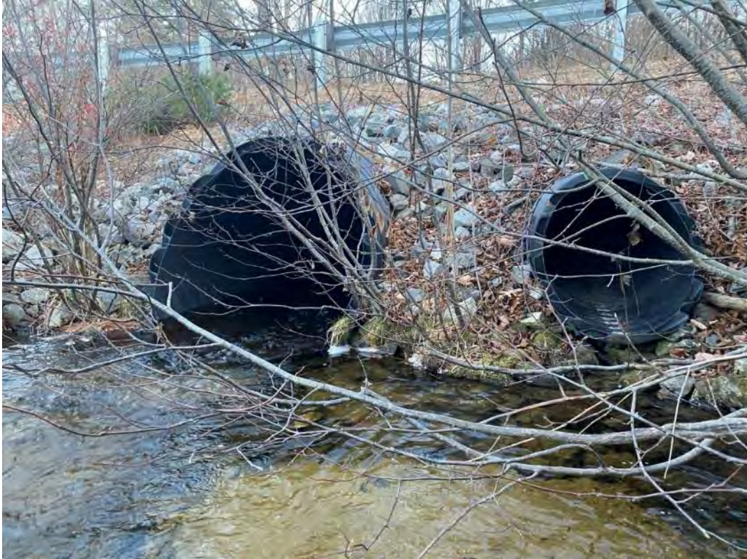
Outlet – 18” and 48” HDPE Culverts (taken May 4, 2023)
