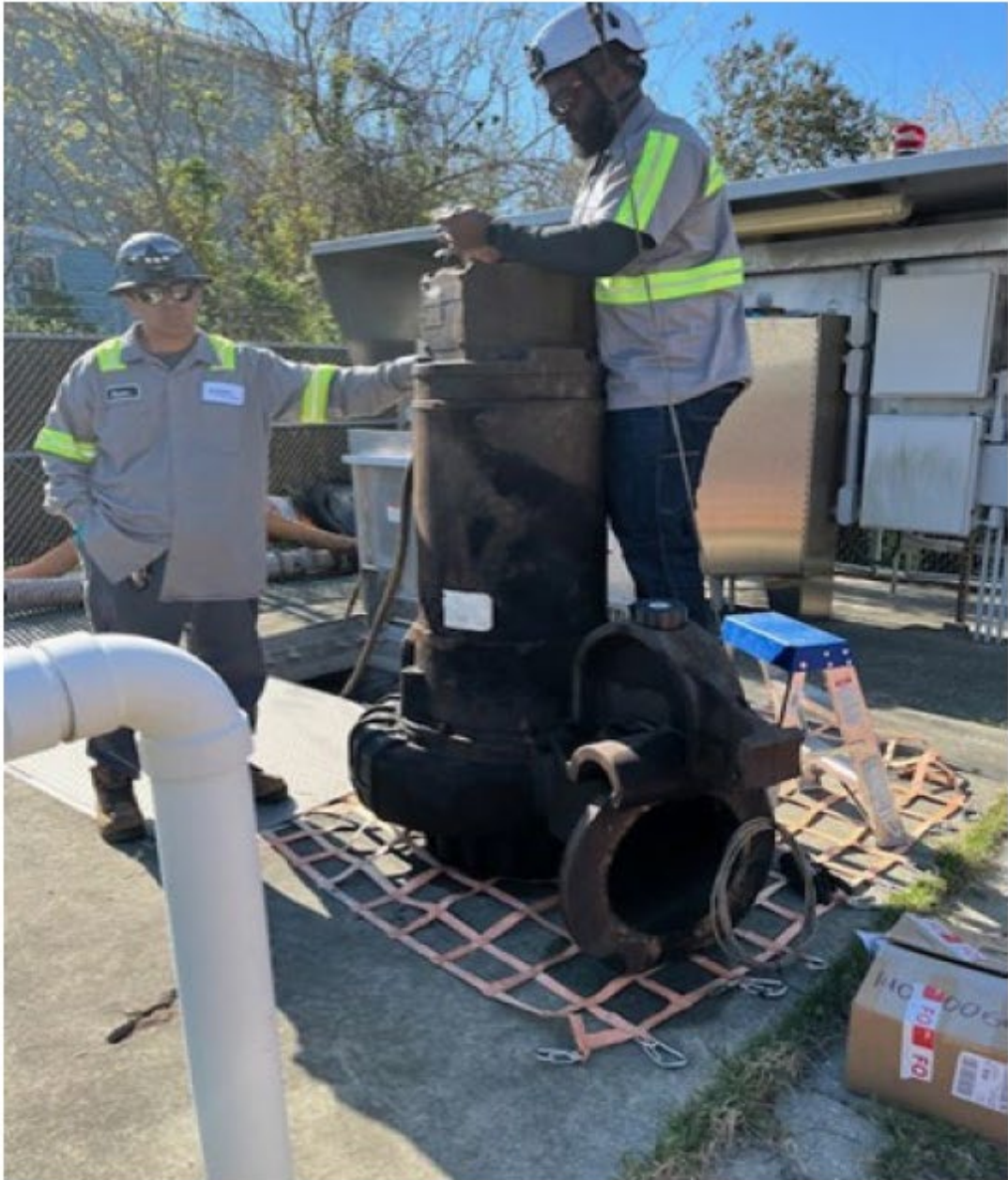
Greenville Ave. pump station received service and an updated alarm panel
