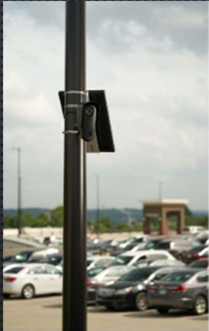
Solar & Existing Pole
