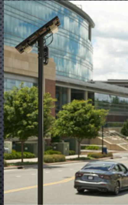
Solar & Flock Pole
