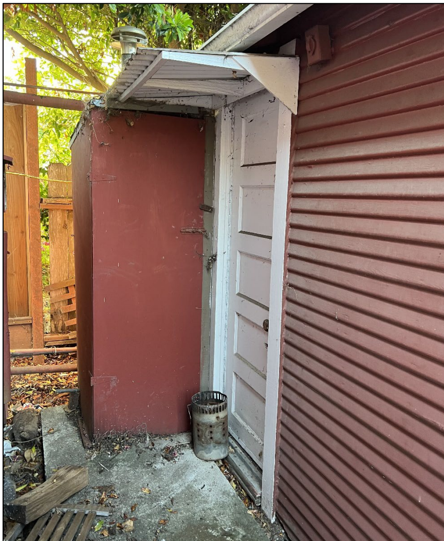
Photograph 11: Detail view of the paneled wood door at the secondary entrance to the storage building. Camera facing south, June 22, 2022.
