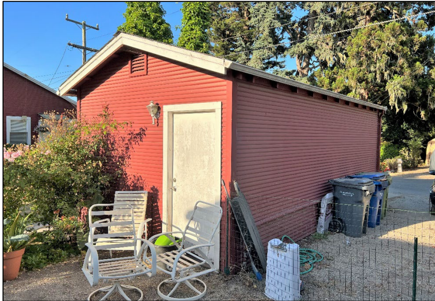
Photograph 7: Garage viewed from the north corner, showing secondary entrance on the northeast gable end of the building and lack of fenestration on the northwest side. Camera facing south, June 22, 2022.
