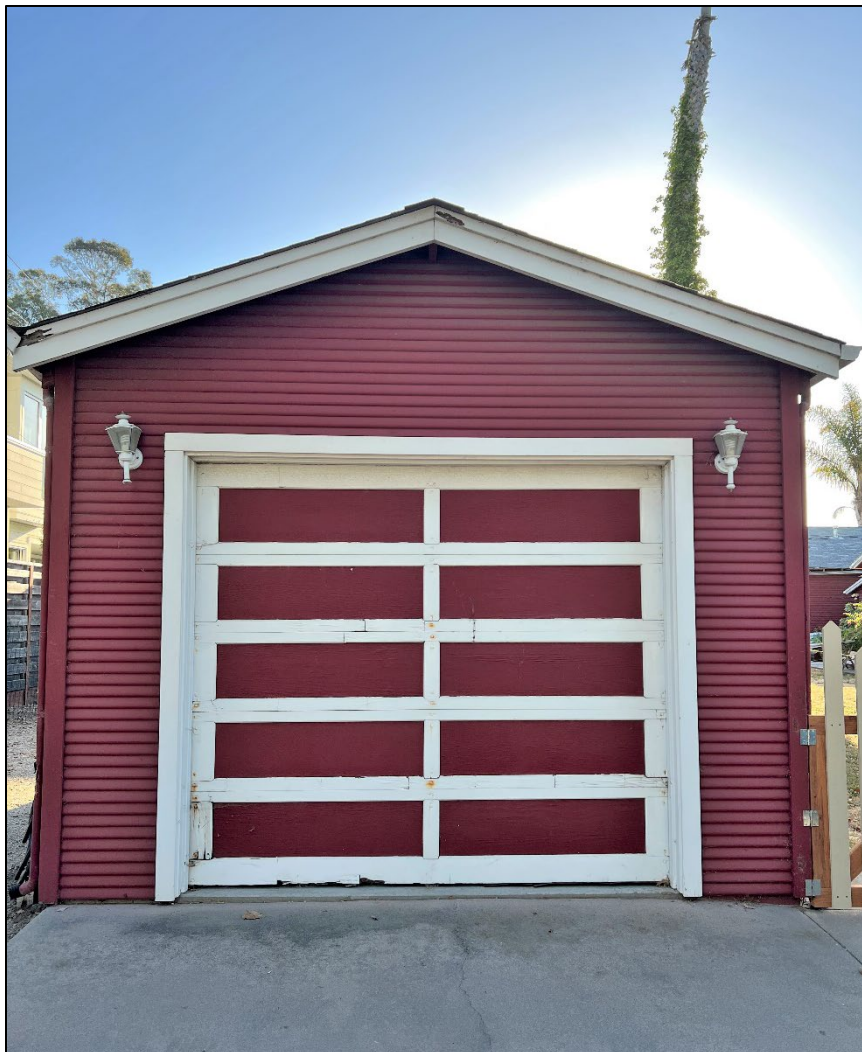
Photograph 6: Southwest façade of the garage, showing tilt-up, paneled wood door. Camera facing northeast, June 22, 2022.
