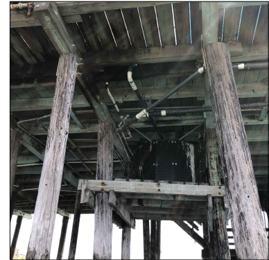
PHOTO 8 UTILITIES AT SEWAGE EJECTOR PUMP
