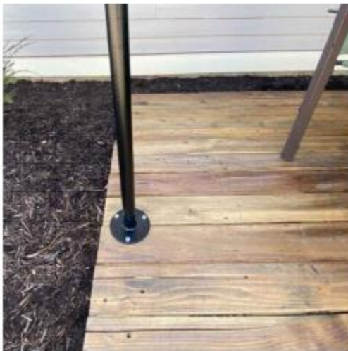
Deck mounted metal poles and LED string lights
