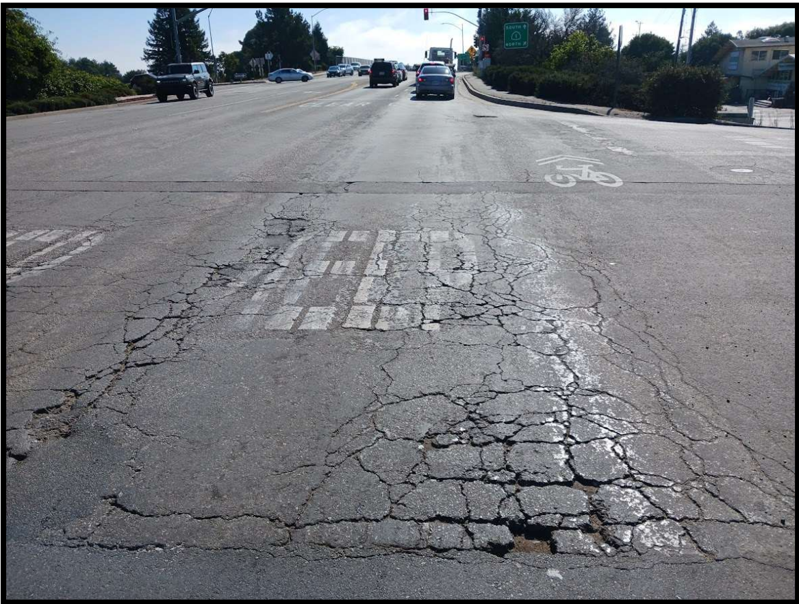
Example of poor pavement condition on 41 st Avenue looking south
