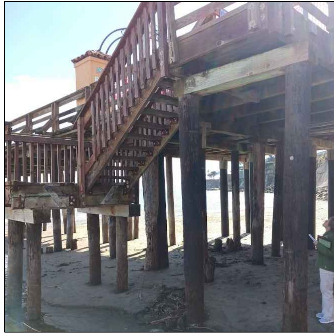
PHOTO 9 STORM DAMAGE AT STAIRS
