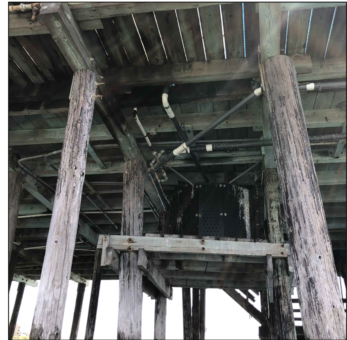
PHOTO 8 UTILITIES AT SEWAGE EJECTOR PUMP
