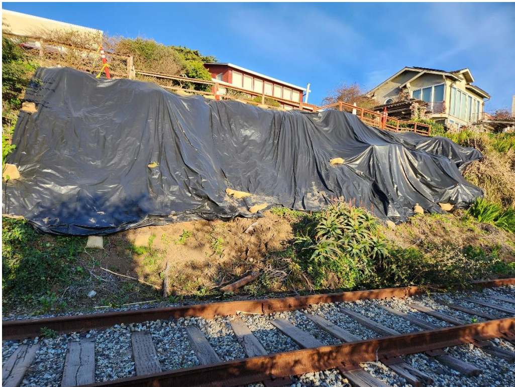
Figure 5. Slope failure adjacent to 1400 and 1410 Prospect Avenue
