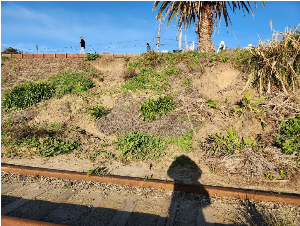
Figure 4. Slope Failures – West
