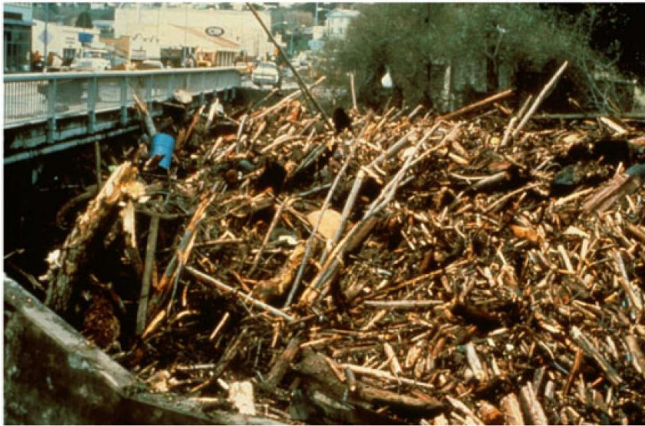
Figure 4. Logjam upstream of Soquel Drive Bridge after January 1982 storm.
