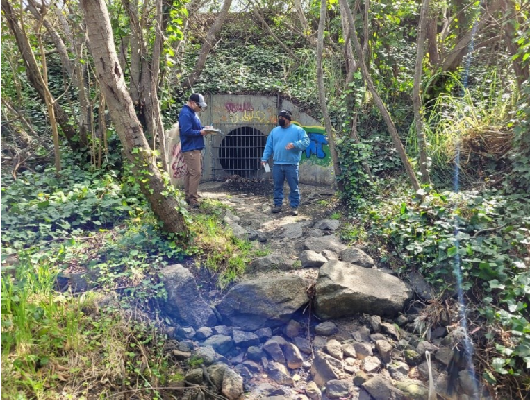
Figure 9. Simpkins Ditch and Outfall with Trash Rack
