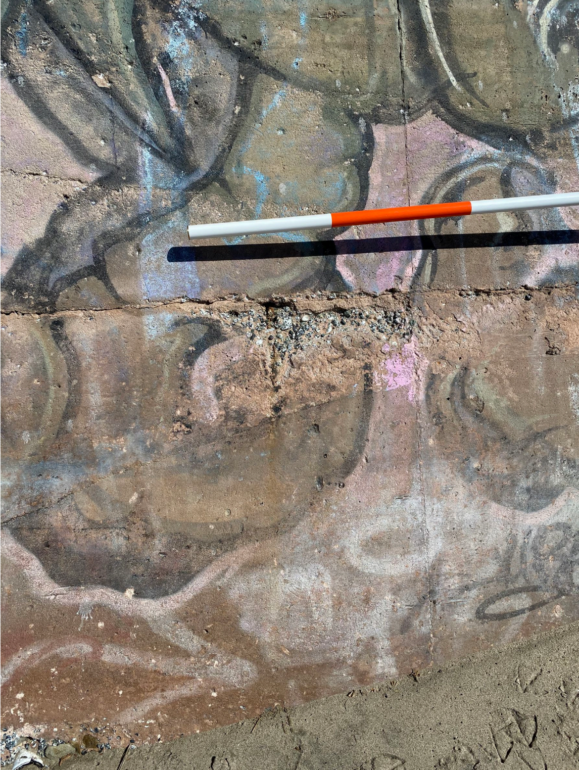
Photo 6: Close up of concrete spalling on bluff toe concrete gravity seawall - 26 May 2020
