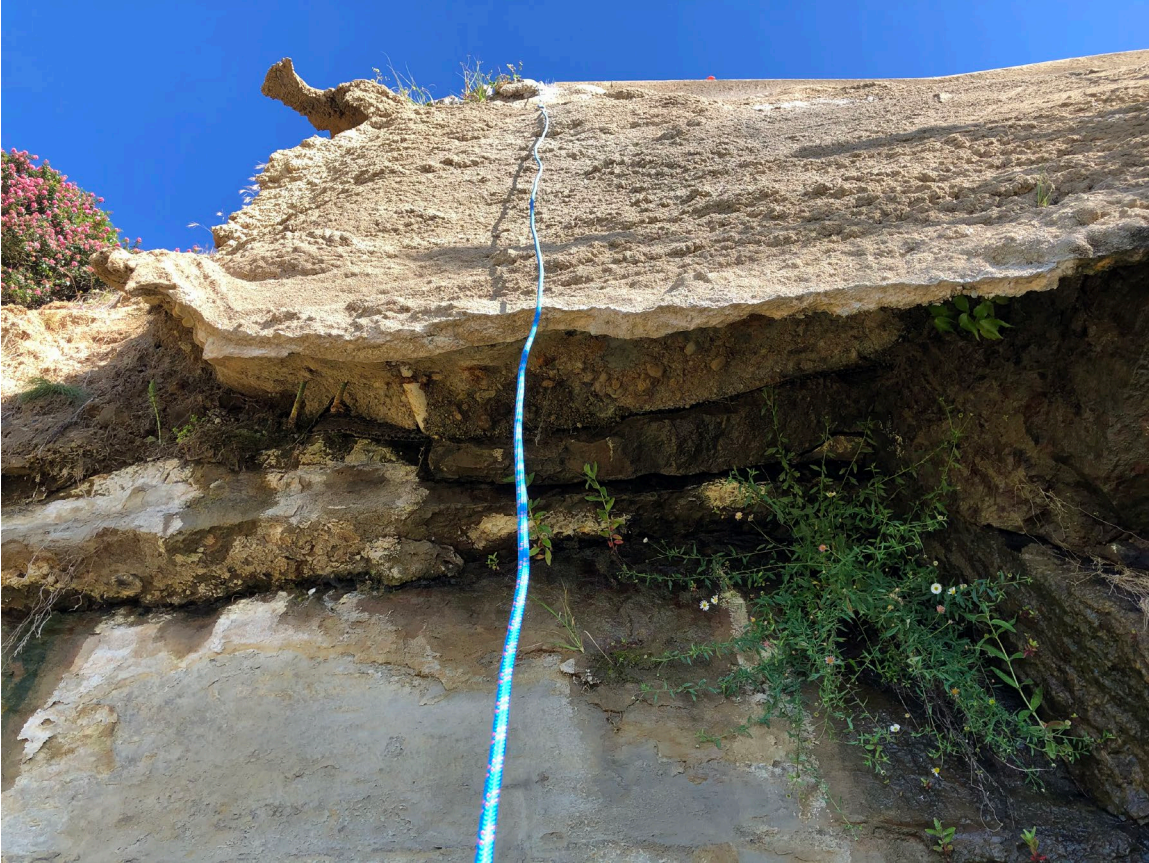
Photo 3: Close up of undermined area in need of repair - 26 May 2020
