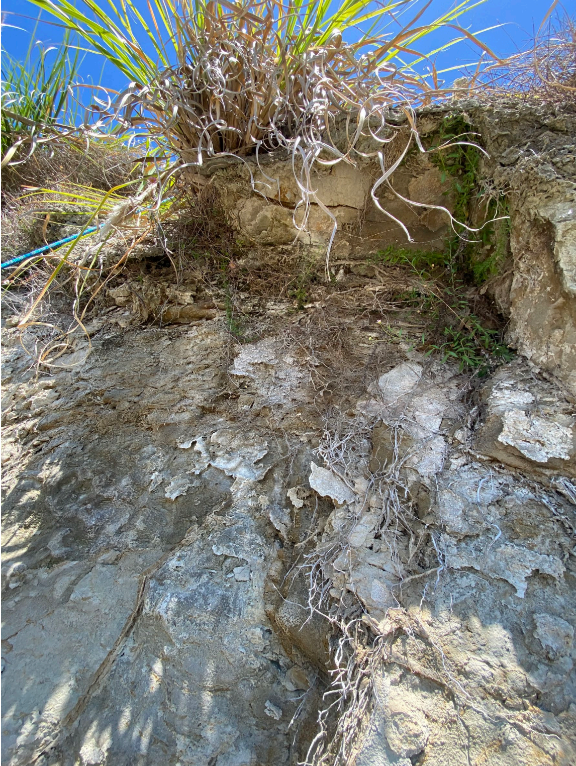
Photo 5: Close up of undermined area in need of repair - 26 May 2020
