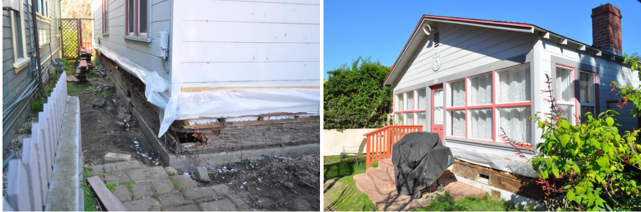
Figures 3 and 4. Left image details the south elevation, showing extensive rot to the sill plate. Right image details the west elevation, showing the deteriorated chimney and rear deck, which was replaced previously.
