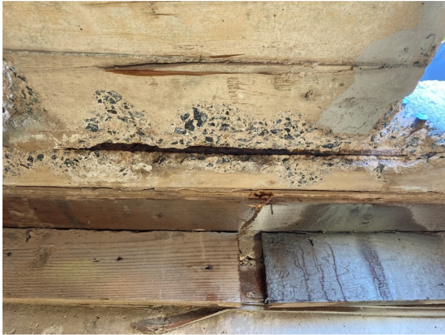
Roadway Deck Soffit Spalls and Reinforcing Corrosion
