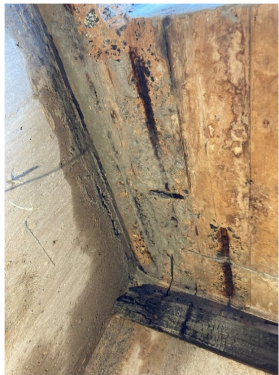
Roadway Deck Soffit Spalls and Corrosion
