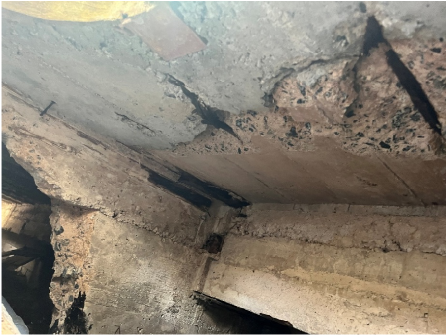
Sidewalk Slab Soffit Spalls and Reinforcing Corrosion
