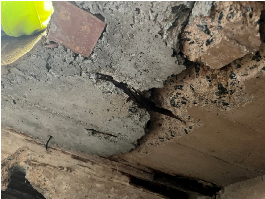
Sidewalk Slab Soffit Spalls and Reinforcing Corrosion
