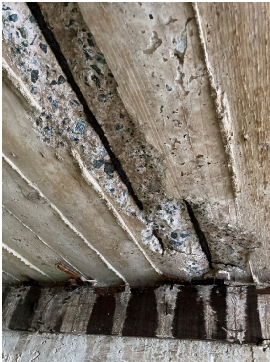
Roadway Deck Soffit Spalls and Corrosion
