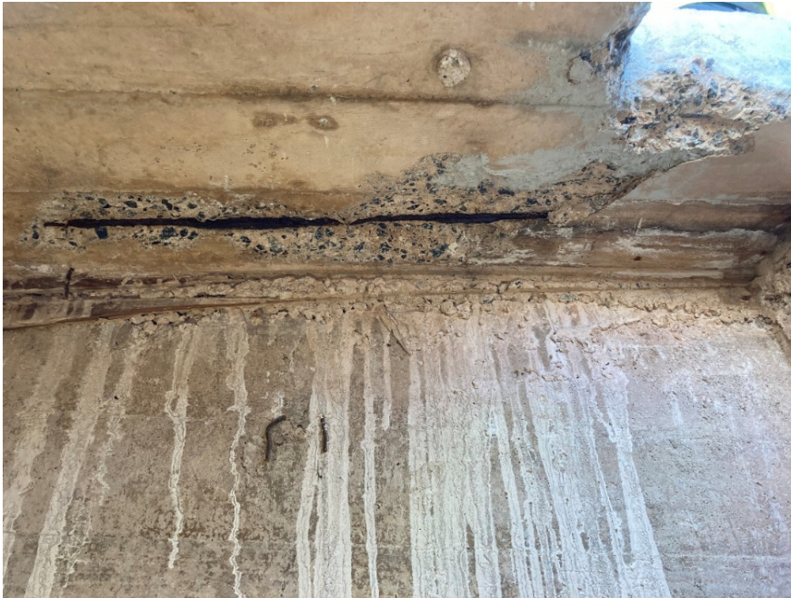
Roadway Deck Soffit Spalls and Reinforcing Corrosion
