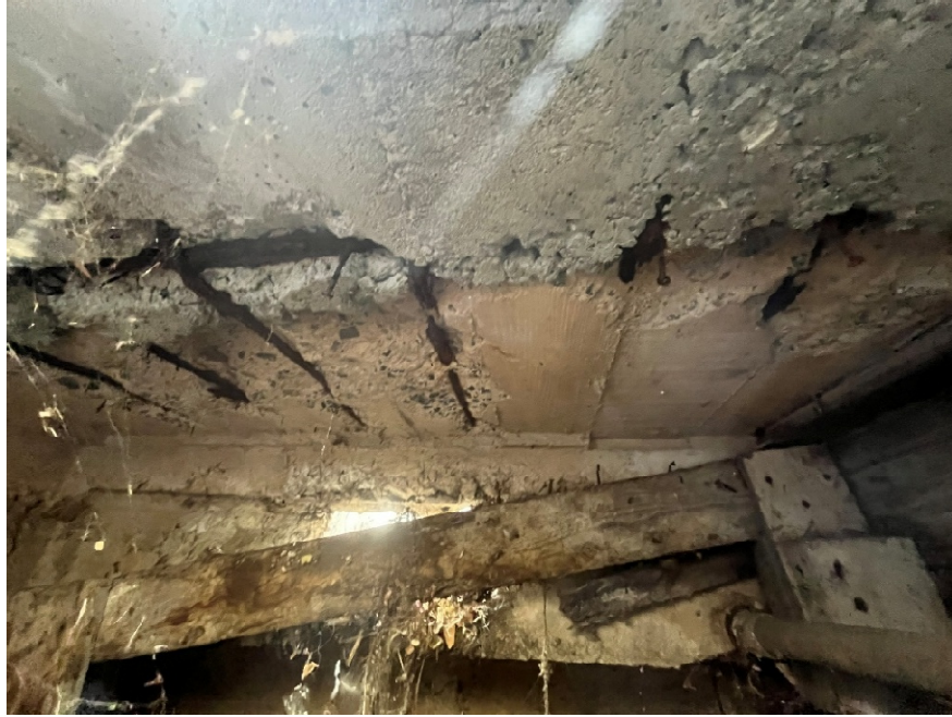
Sidewalk Slab Soffit Spalls and Reinforcing Corrosion
