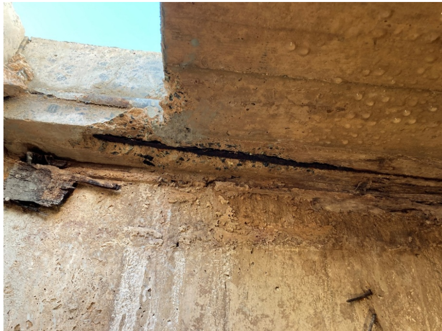
Roadway Deck Soffit Spalls and Reinforcing Corrosion
