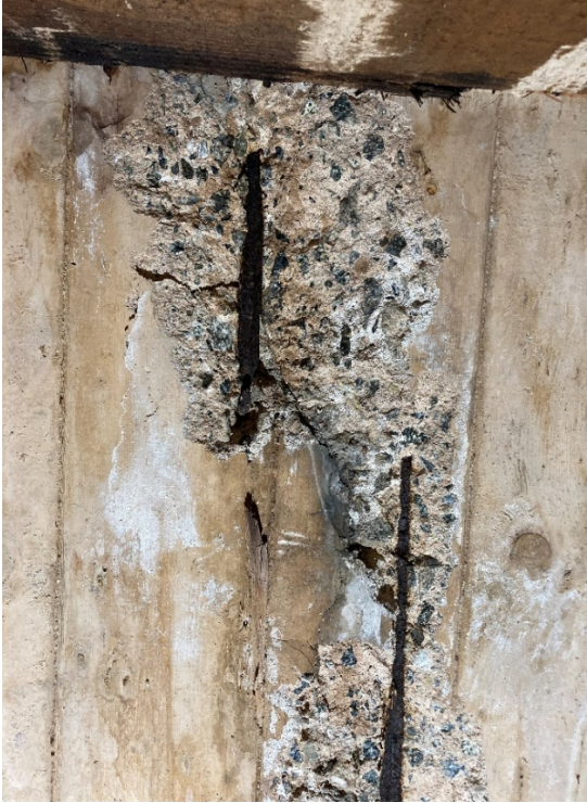
Roadway Deck Soffit Spalls and Reinforcing Corrosion
