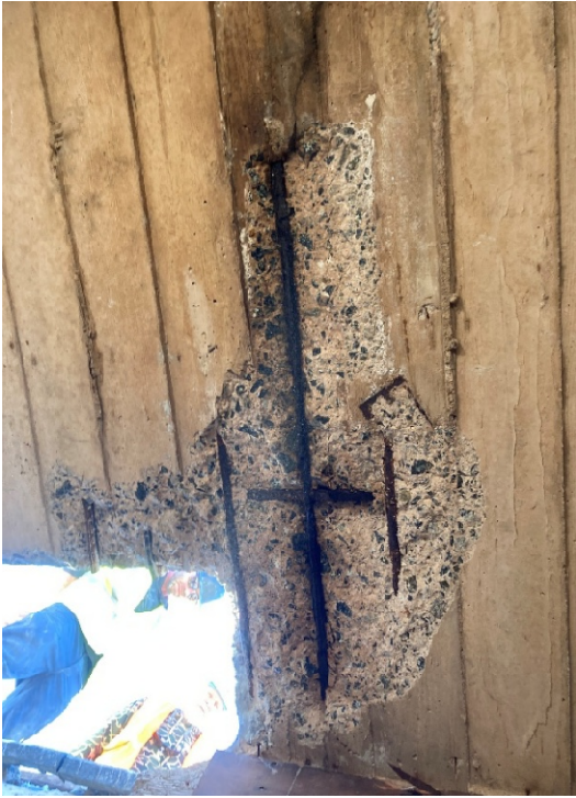
Deck Soffit Spalls and Reinforcing Corrosion
