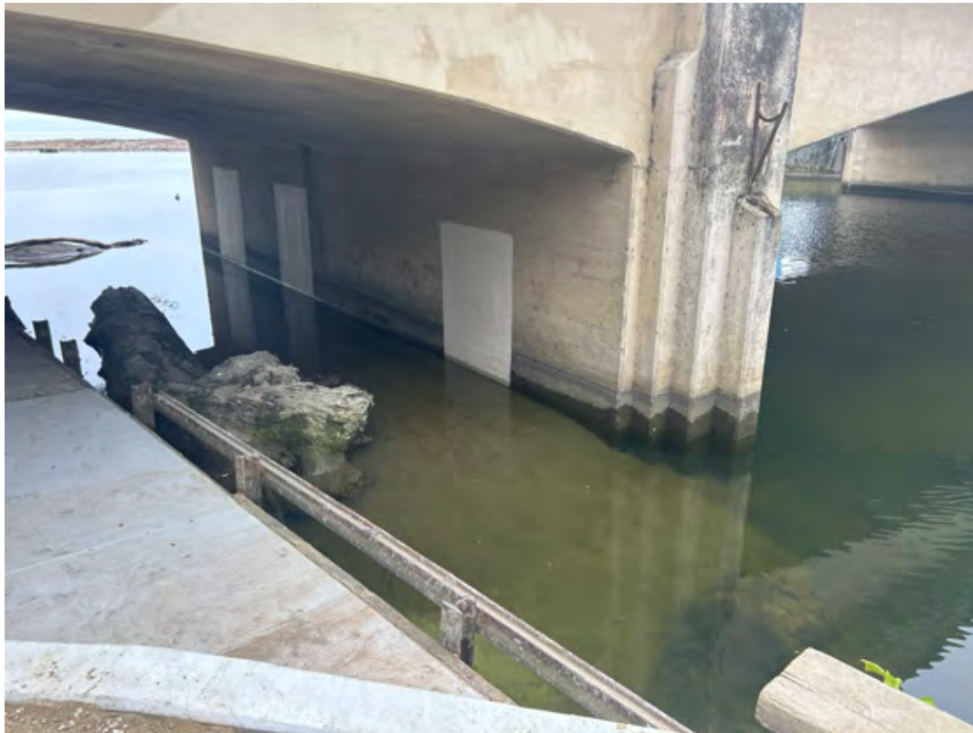
Photo 2. OHWM on the south pier of Stockton Bridge (5/14/2024).
