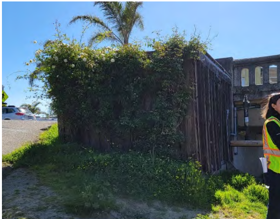
Figure 9 Existing Pump House
