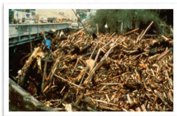
Figure: 1982 Debris Accumulation upstream of Soquel Drive Bridge.
