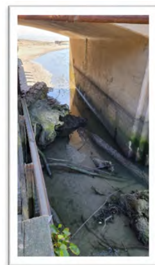
Figure: Debris Accumulation in Eastern Span of Stockton Avenue Bridge
