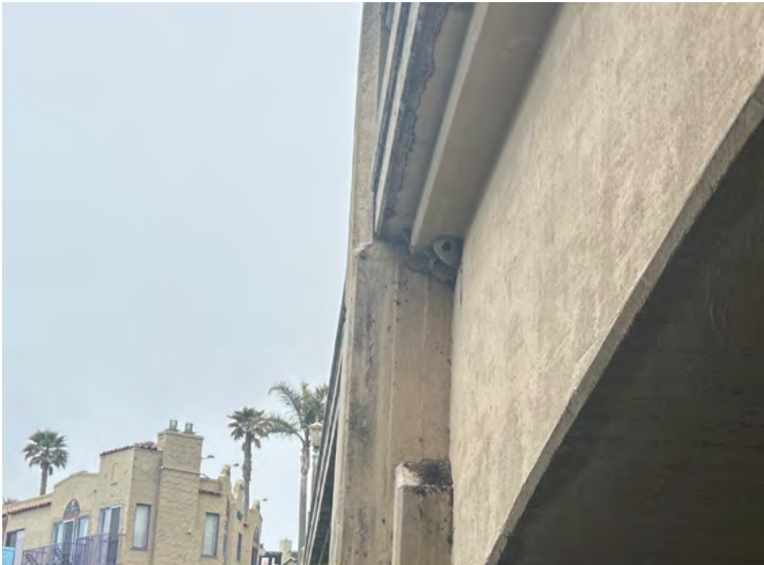
Photo 4. Swallow nests observed on the underside of Stockton Bridge deck
