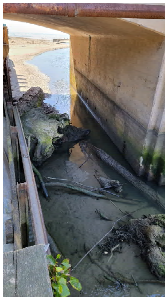
Figure 4 Debris Accumulation in Southern Span
