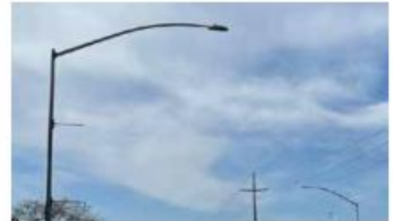
Caltrans standard cobra head for vehicular lighting. (Photo by: SWA)
