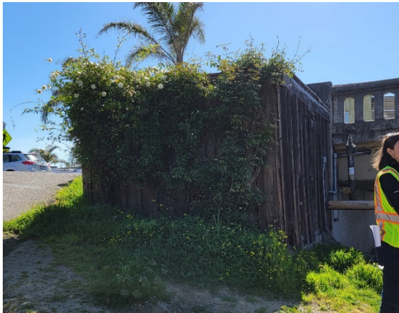
Figure 9 Existing Pump House
