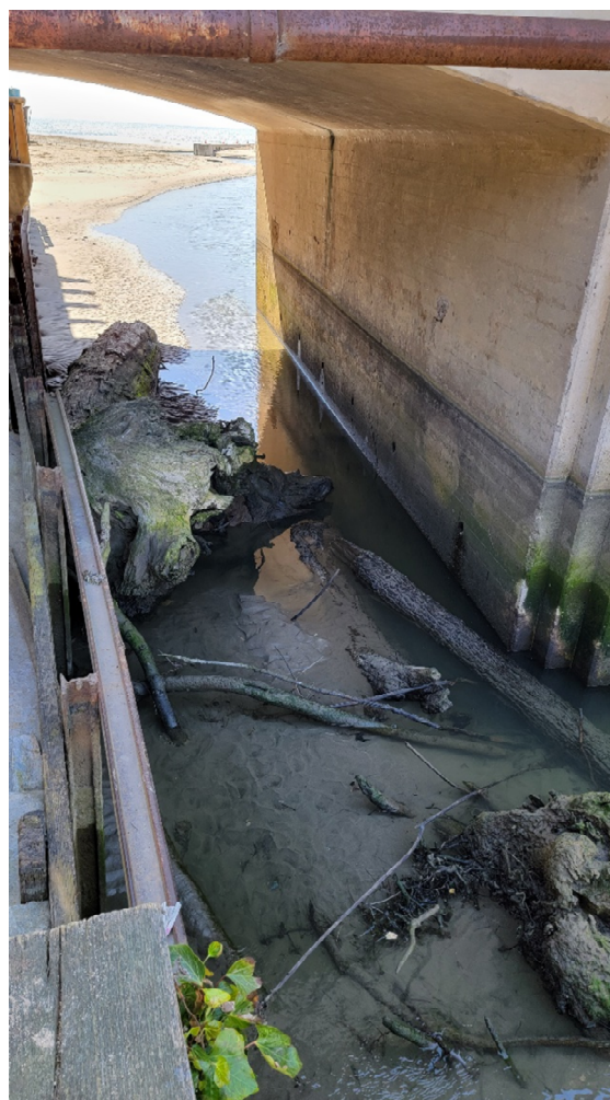
Figure 4 Debris Accumulation in Southern Span
