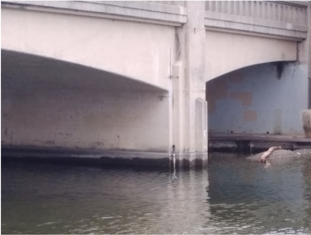
Photo 3. OCHM on the north pier of Stockton Bridge (5/14/2024).
