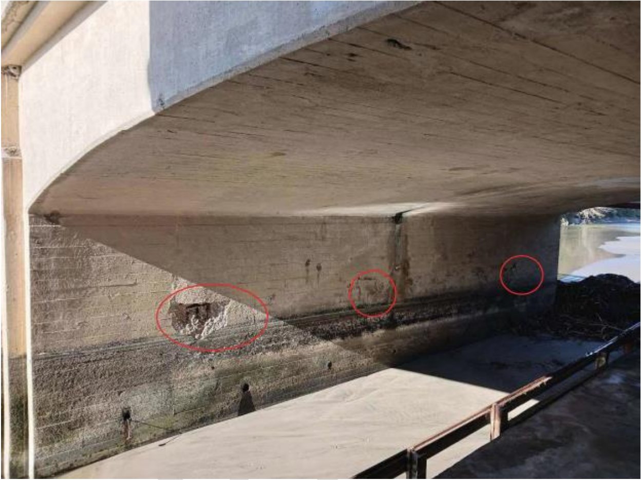
Figure 2: East Pier Wall During Very Low Tide with Spalled Areas Circled in Red
