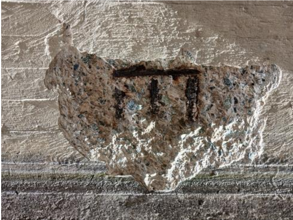
Figure 6: Close-up of Exposed Rebar Under Spall on East Pier Wall
