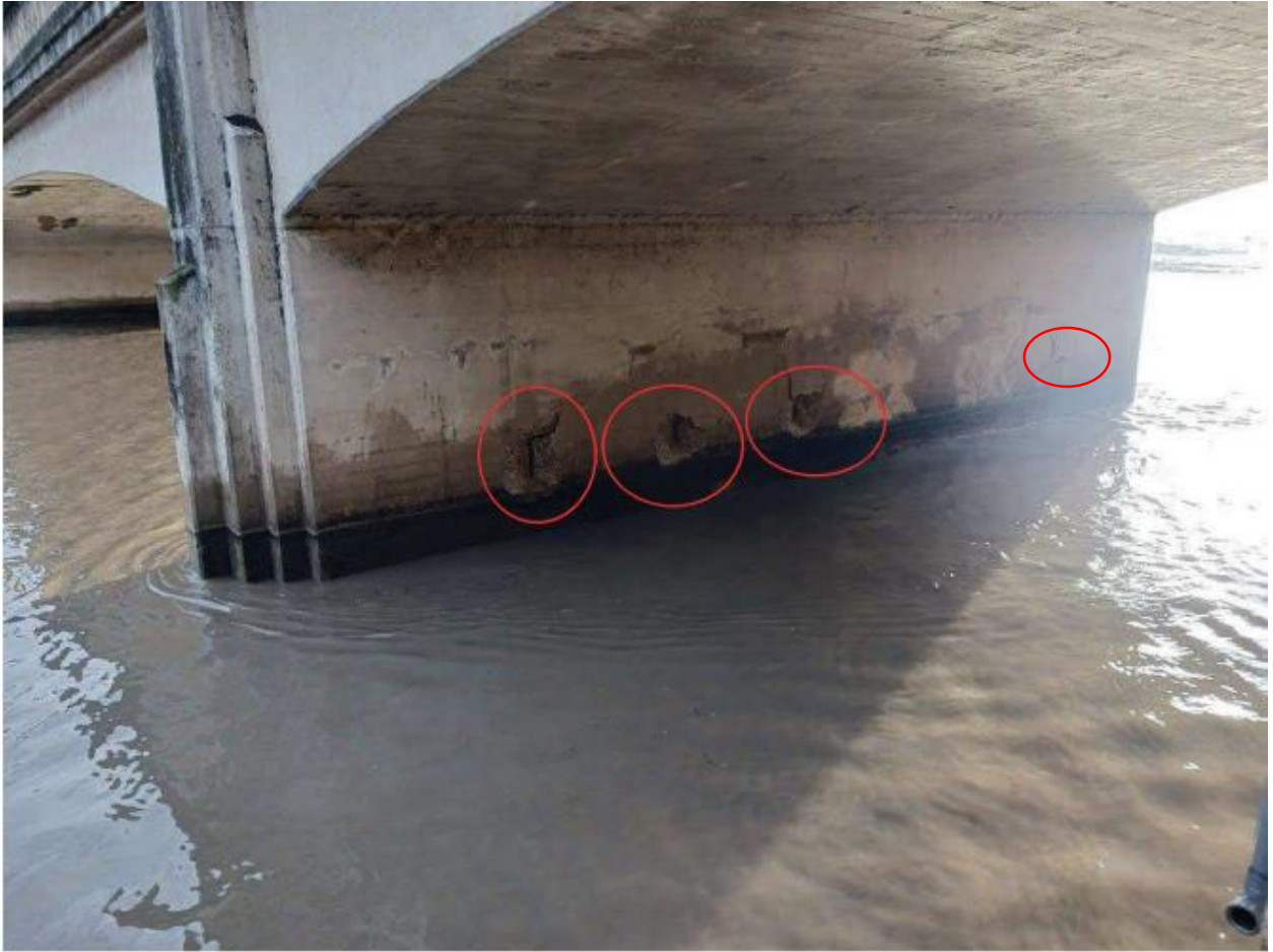
Figure 3: West Pier Wall in Post Storm Condition with Spalled Areas Circled in Red
