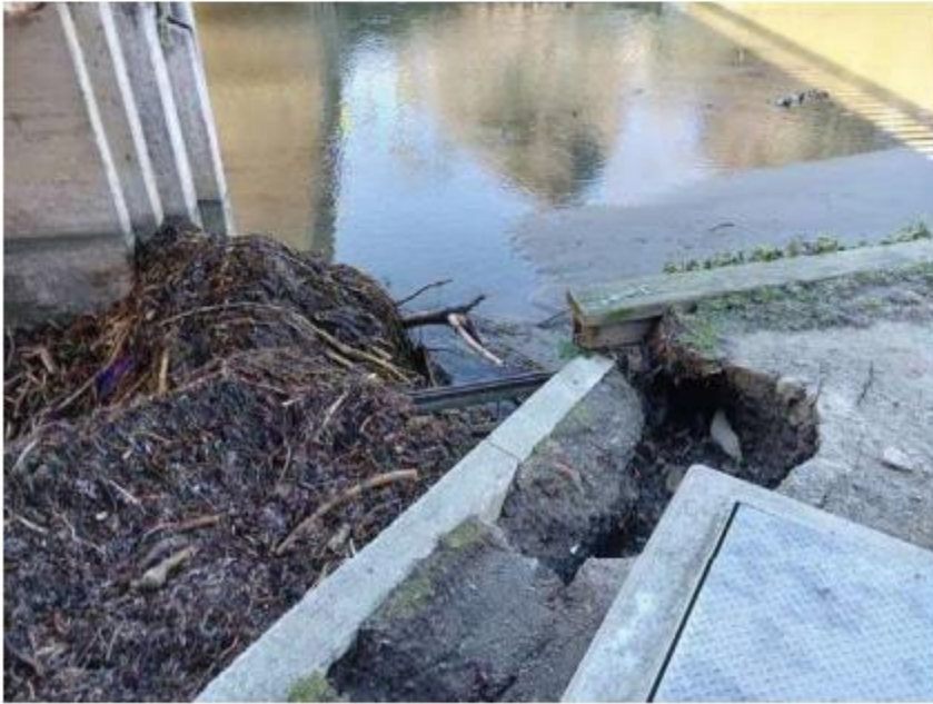
Figure 4 & 5: Retaining Wall During Very Low Tide Showing Debris Accumulation
