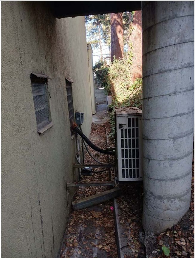
Location B – Electrical Room
