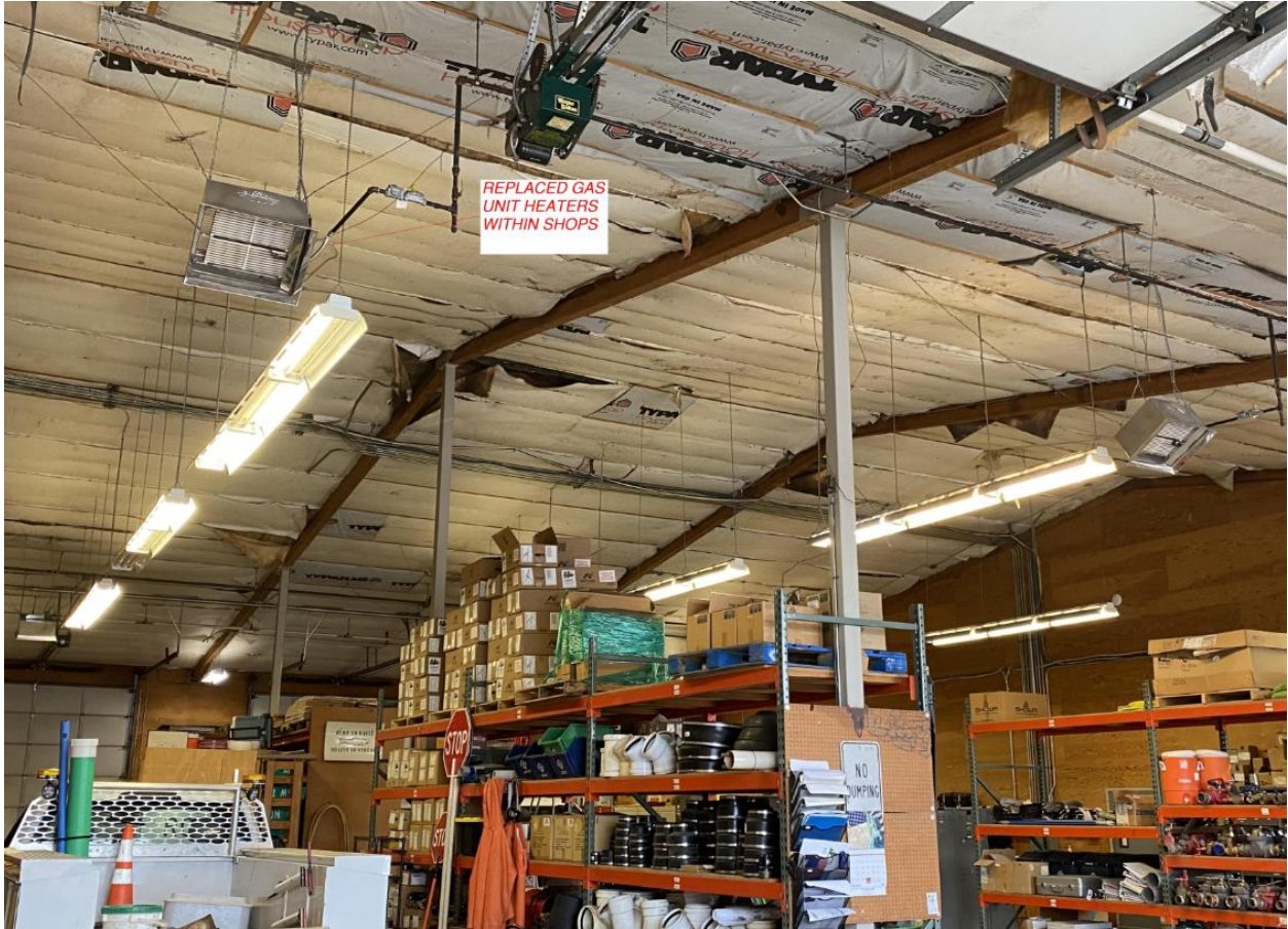
New unit heaters within maintenance garage
