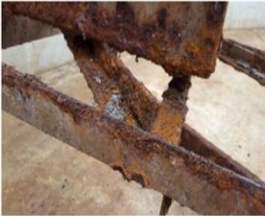
Figures 3-5: Corroded Metal in Primary Clarifier Basin
