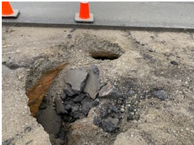
Figure 1. Sinkhole under Endicott St.
