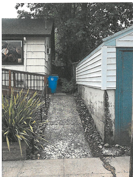
Encroaching garage to northwest of west property line
