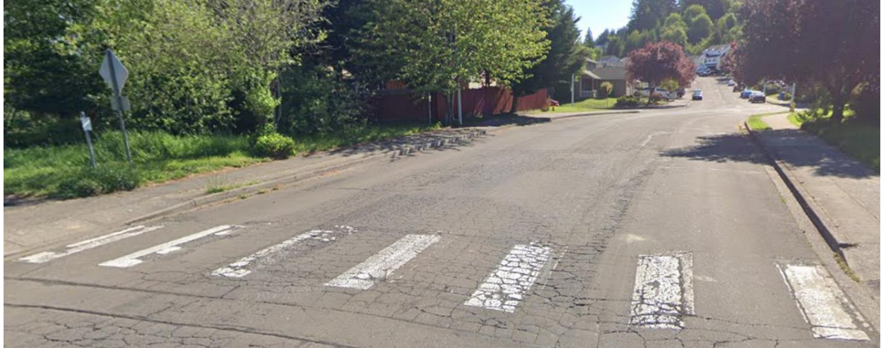
Figure 2: Photo from 2023 showing Pavement Failure East of NW Knapp LN
