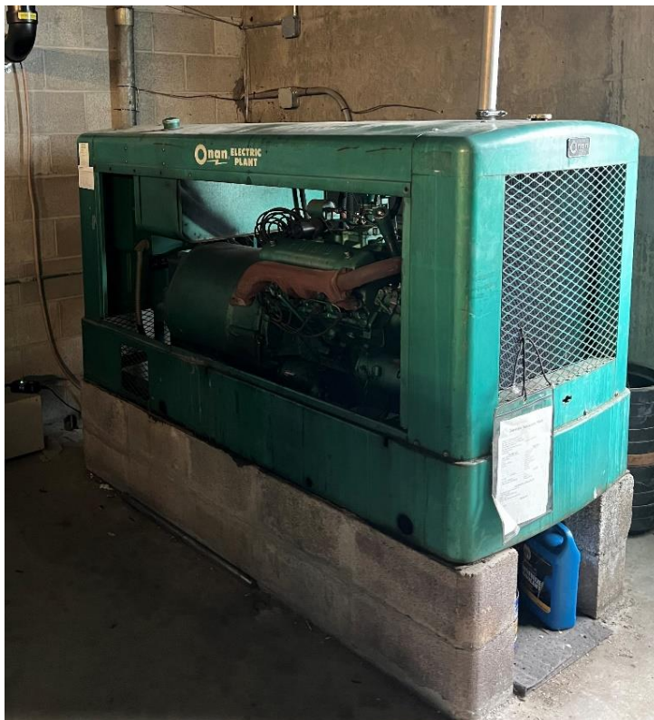
Figure 1: Existing Generator to be replaced (1967 Onan 40-KW Natural Gas Generator)
