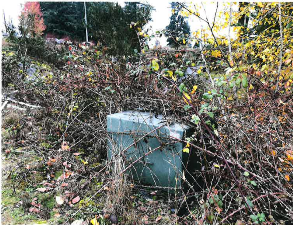
Photo 2 – Pad mounted transformer in brush on southeast side of parking area
