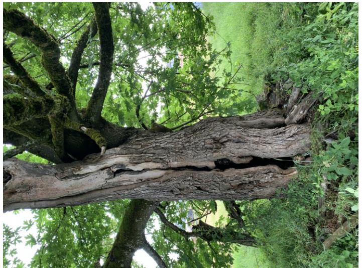
Tree#5 South crack/bole splitting
