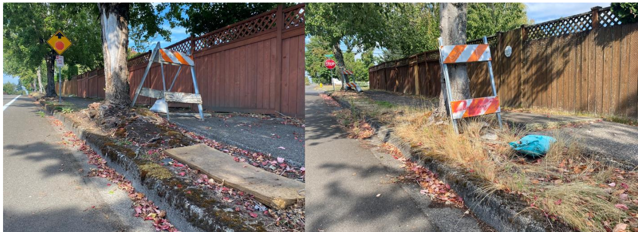
Figure 1 & 2: Sidewalk conditions sample
