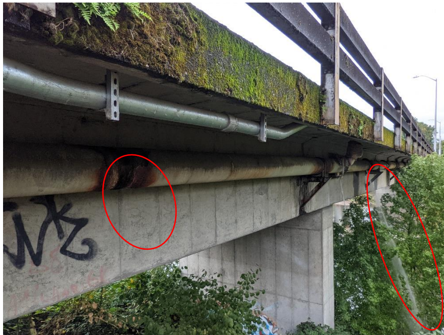
Figure 1: SE 6 th Washougal River Bridge: Leak and Corrosion at Joints.
