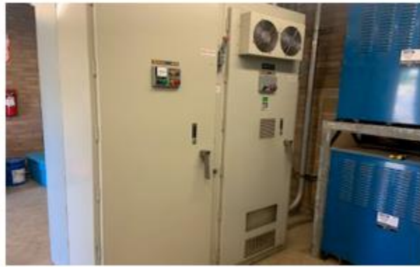
Fig 2: Variable Frequency Drive Panel
