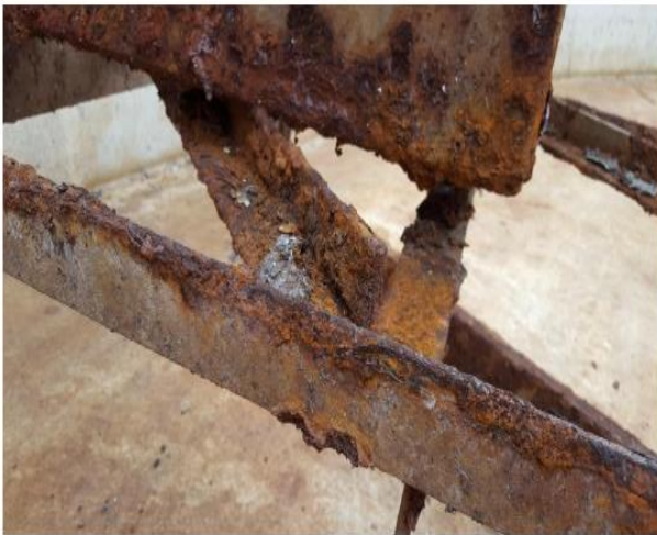
Figures 3-5: Corroded Metal in Primary Clarifier Basin
