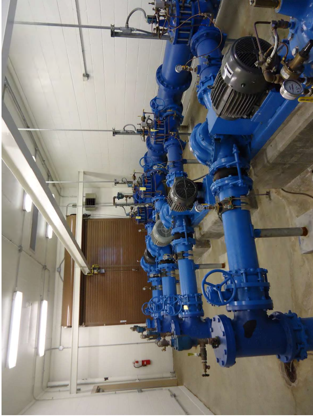
UPPER PRUNE HILL BOOSTER PUMP STATION
