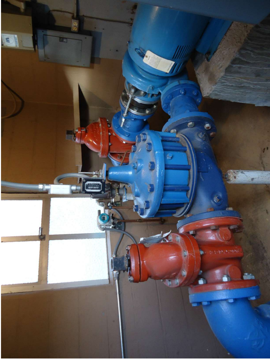
FOREST HOME BOOSTER PUMP STATION
