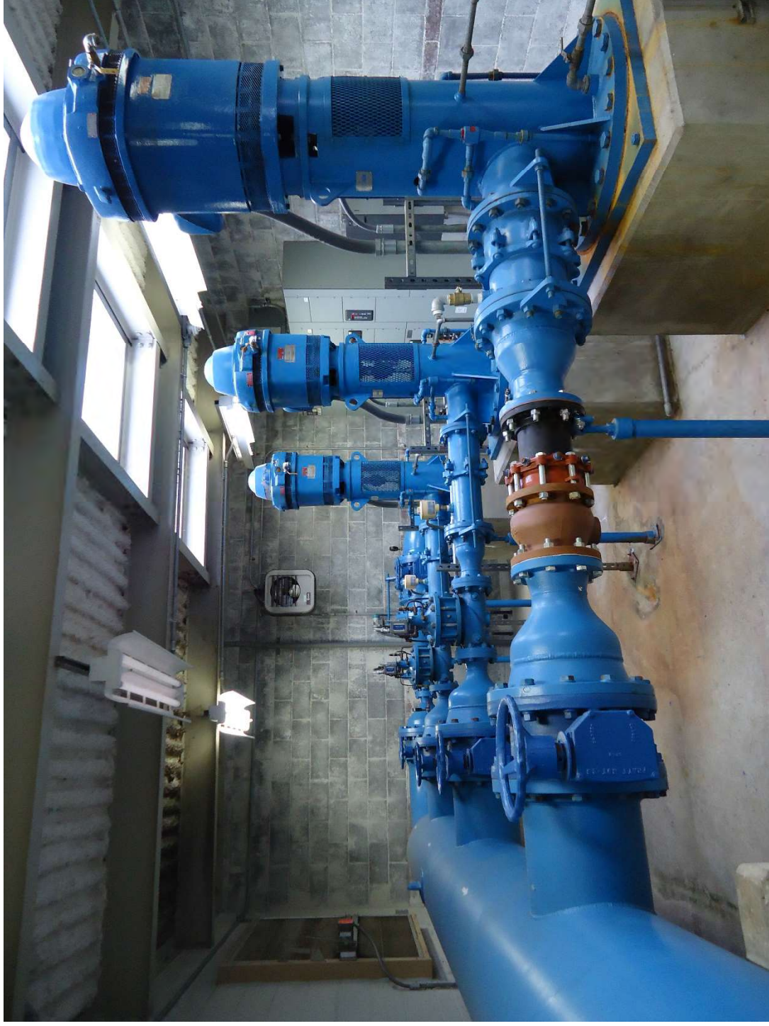
LACAMAS BOOSTER PUMP STATION
