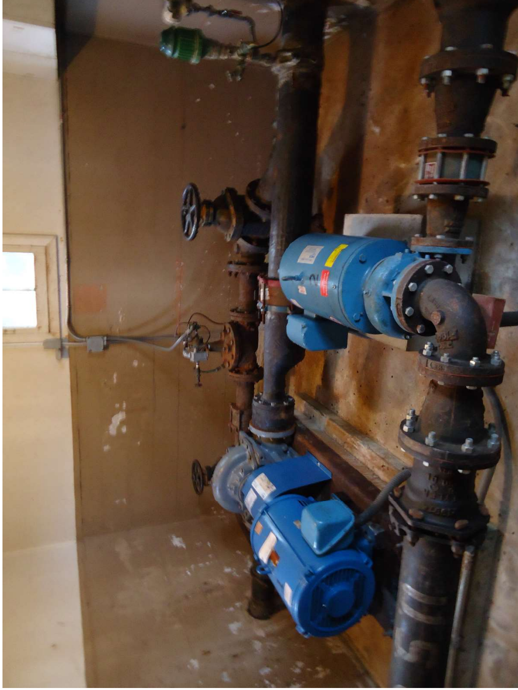
BUTLER BOOSTER PUMP STATION
