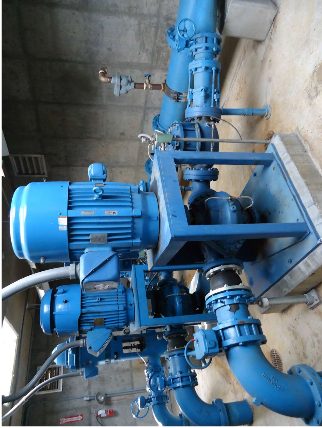
LOWER PRUNE HILL BOOSTER PUMP STATION
